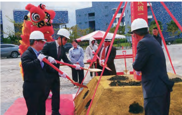
NIAR President Hung-Yin Tsai presides over the groundbreaking ceremony, marking the start of the project.
