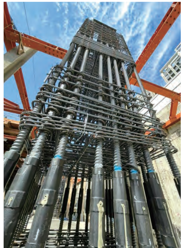
Construction using prefabricated rebar cages with SA-grade mechanical couplers. (Image source :Toong Rong Iron & Steel Enterprise Co., Ltd. (Taiwan)).
